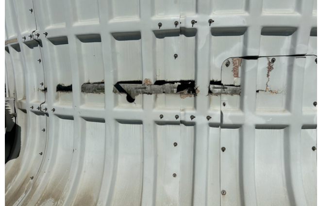
Fig 1. Damage from freewheeling fan
